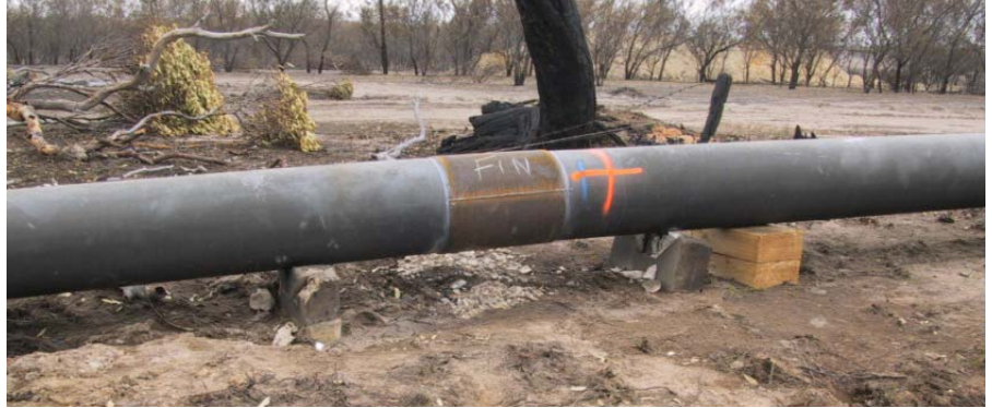
Steel repair band welded around failed joint. Pipe supported on temporary timber blocks as concrete supports were damaged
