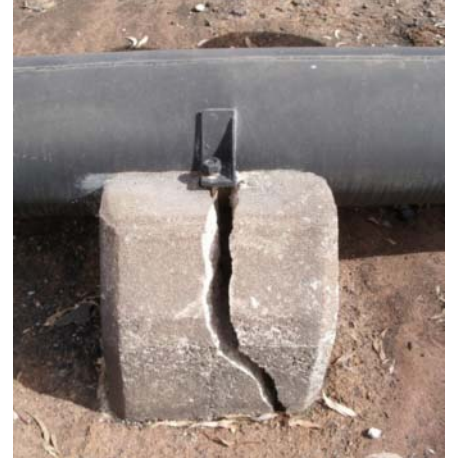
Concrete thrust block split on each side of hold down bolt
