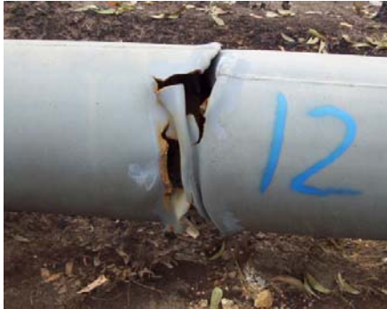
Excessive expansion caused the pipe to concertina and fail at a welded joint
