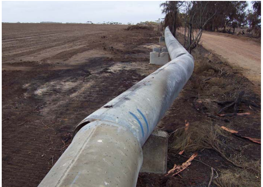
Expansion beyond design limits resulted in the pipe lifting off of the supports, bending and breaking at a welded joint
