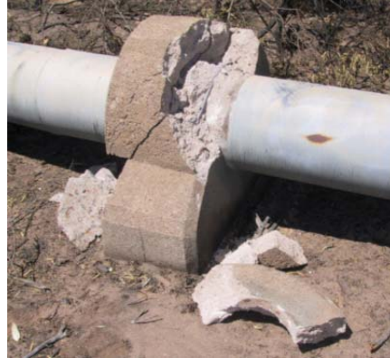
Cracked and spalled concrete thrust block
