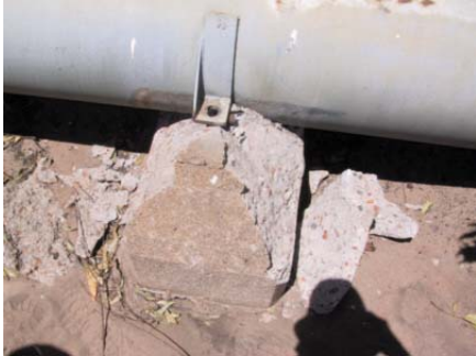
Spalled concrete thrust block with failed anchor bolt
